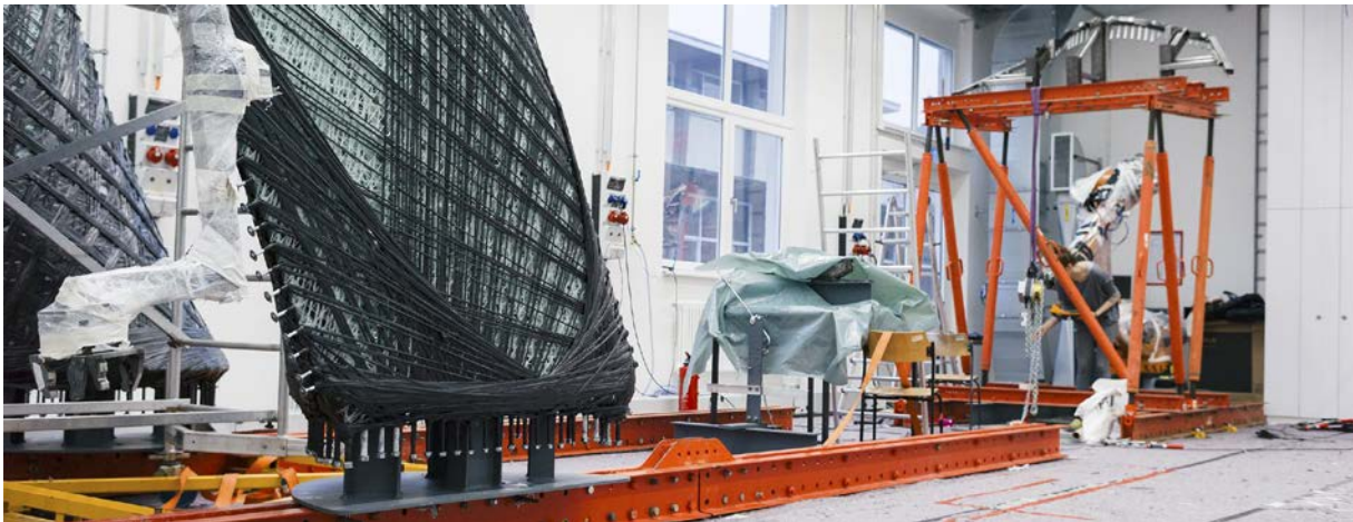
Figure 8: Formwork system of the cantilever (left to right): portal frame and permanent part of the structure, temporary tip frame with push-pull props and steel extension
